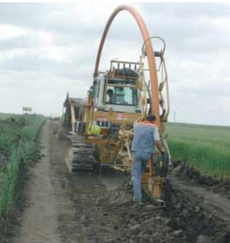
Reduced soil damage and faster laying through the new ploughing process for gas pipeline installation.
