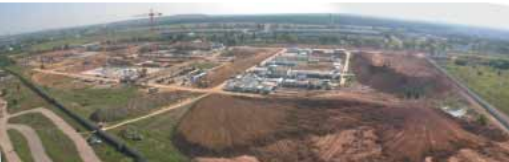
WTE has already made considerable progress with the construction work on the South-West Moscow drinking water plant.
