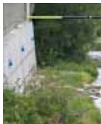
In Baden, the embankment wall of the neighbouring River Schwechat was also appropriately sealed.
