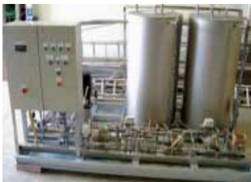
The new washing system for fully automatic cleaning of the condenser at the Theiss power station.
