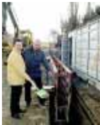
In Stockerau watertight walls ensure the lasting decontamination of the former gasworks site.
