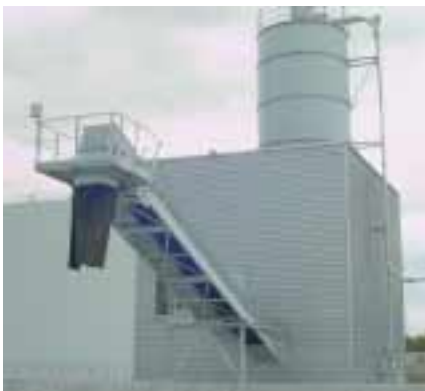
The latest flue gas cleaning systems provide a reduction in emissions from the Theiss power station.
