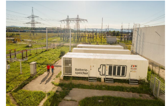
BESS expansion & flexibility management 300 MW storage capacity by 2030
