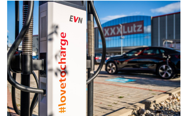
EV charging infrastructure Ongoing expansion of charging points
