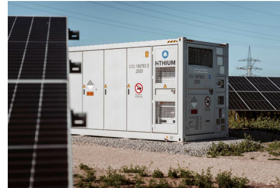
PV panels & battery
