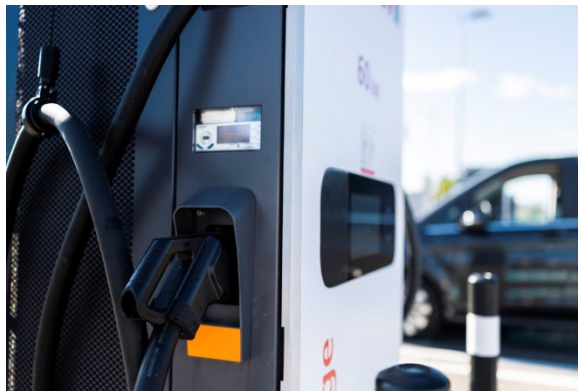
EV charging backend
